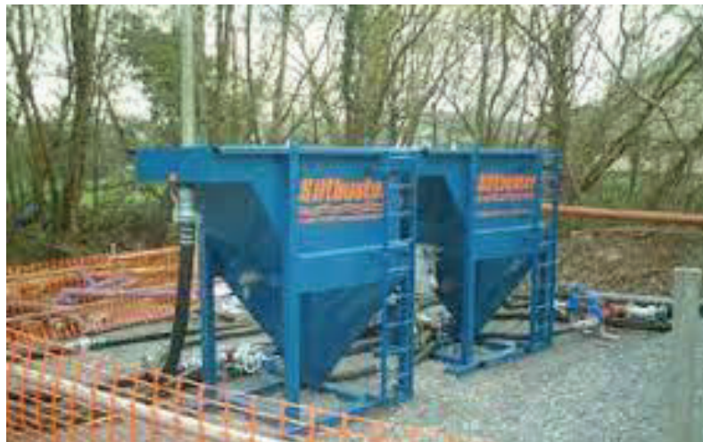
Figure 4.3: Settlement Tank, silt buster lamella settlement tanks ( https://www.siltbuster.co.uk )
